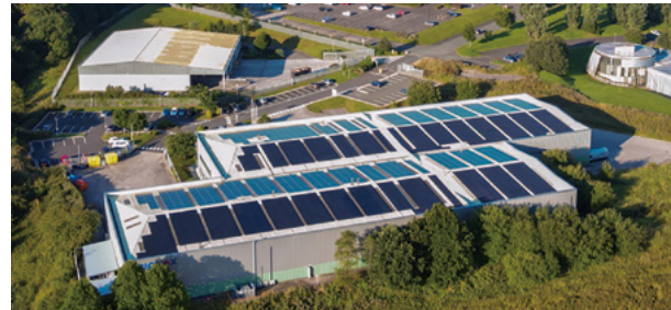
Solar panels in the UK
