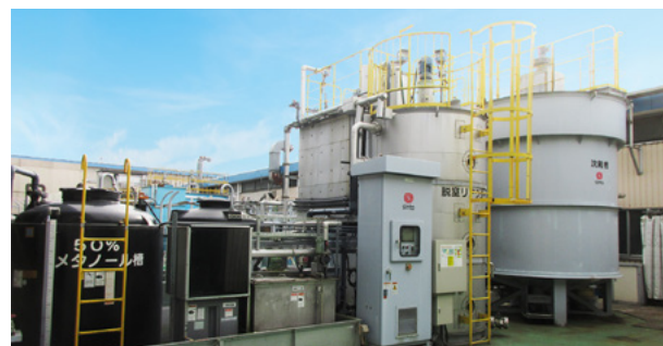
Moka Plant: biological denitrification wastewater treatment
